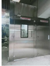
Clean Room Air Shower
